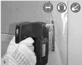
5 Make the opening. NOTE: Load Bearing elements must not be weakened! IMPORTANT: follow the safe working notes on p.35.
