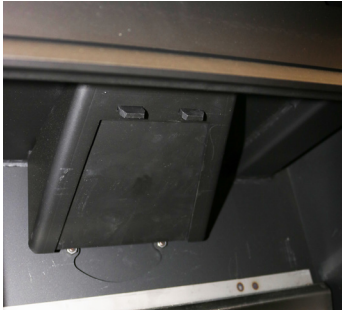
1. The upper steel baffle sits in a bolt-up housing at the top of the inside of the stove
